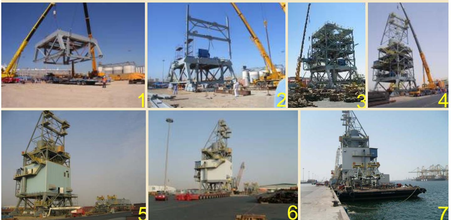
SOHAR ALUMINIUM PROJECT 800 t/h ship unloader 8
