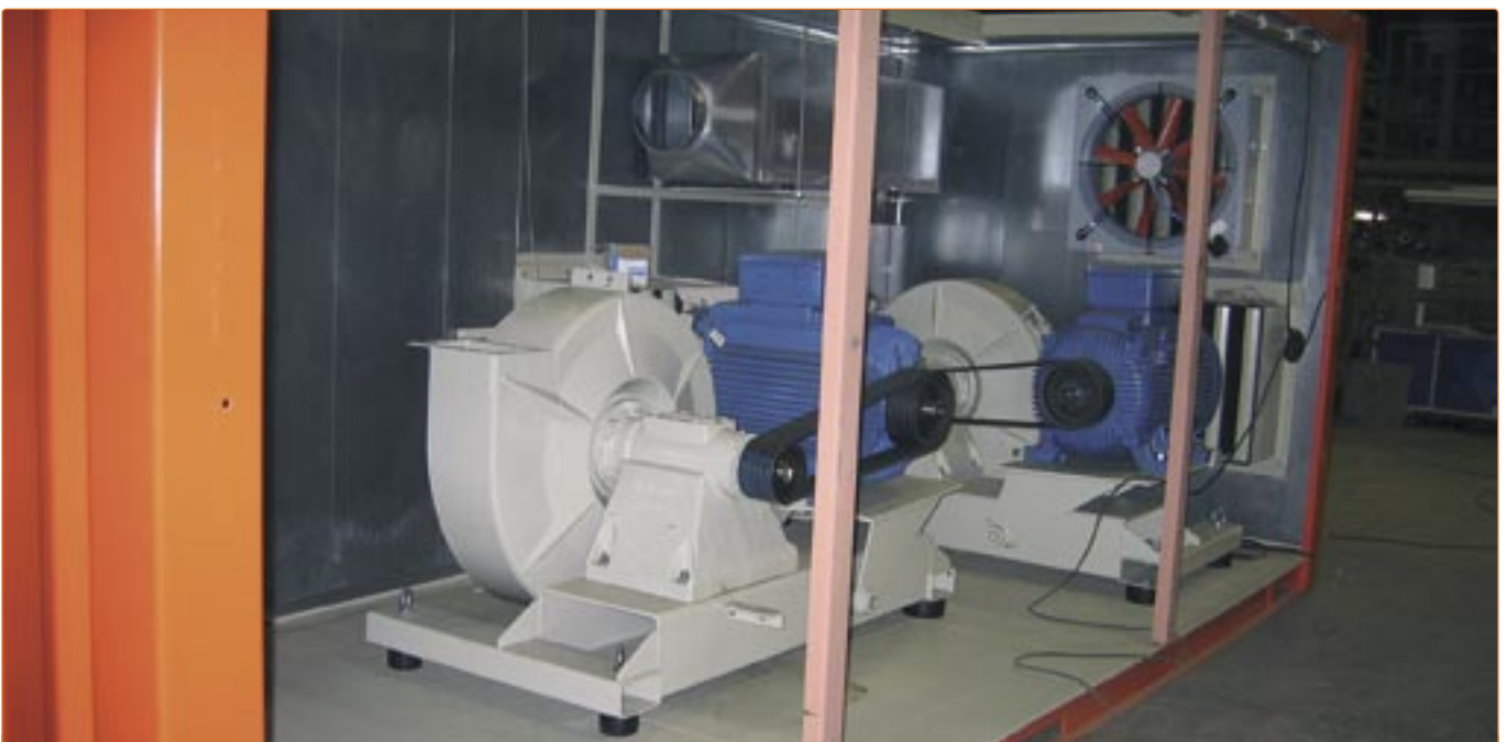
Figure 5. Turbo blower station.
